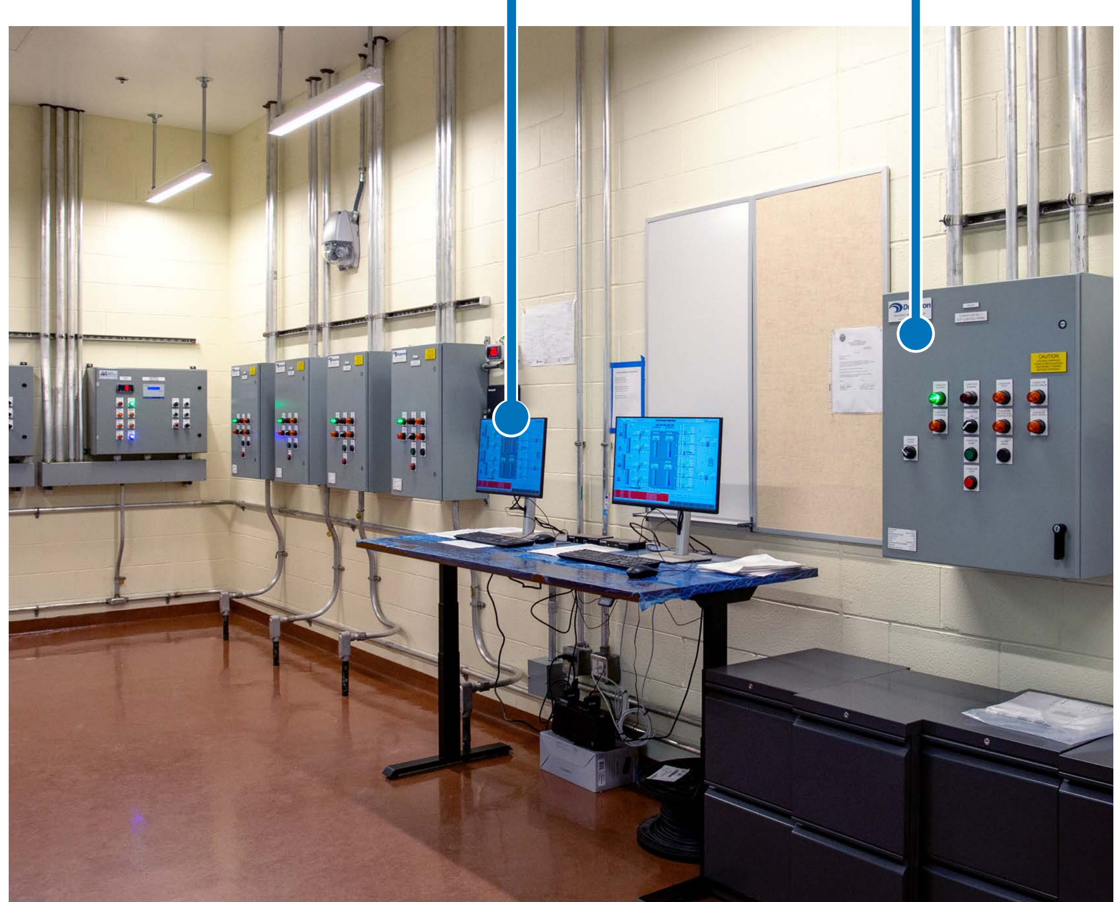
New station's control room
