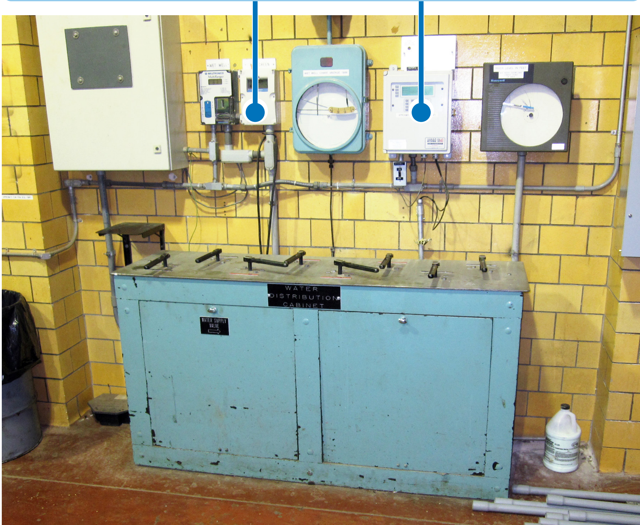
Old station's control room
