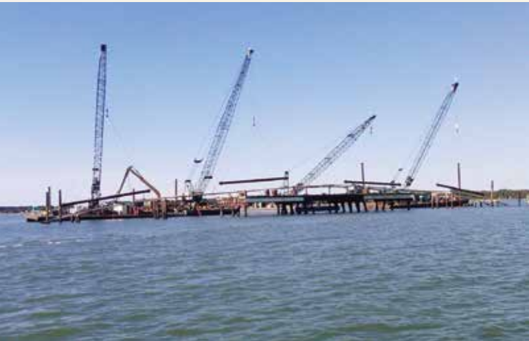
Overboarding pipe from fixed platforms for twin 17,000-foot HDD crossing of York River Power transmission project
