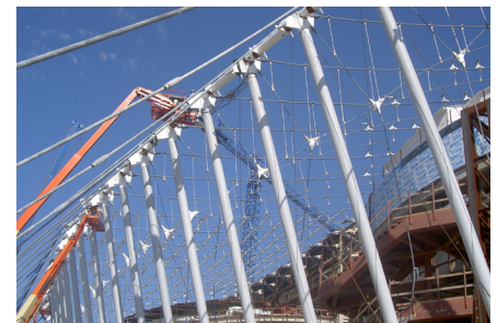
Grand lobby structural cable system
